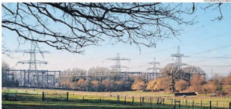
Land west of the Lovedean substation, seen here from the north, has been earmarked by Aquind for a converter station.
